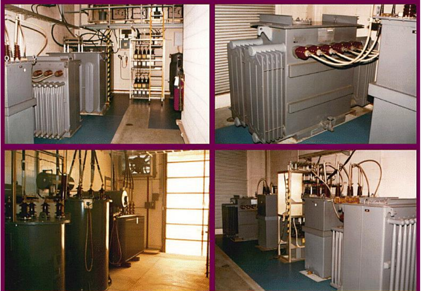
VOA - Views of Transmitter Power Supply and Modulation Components.
