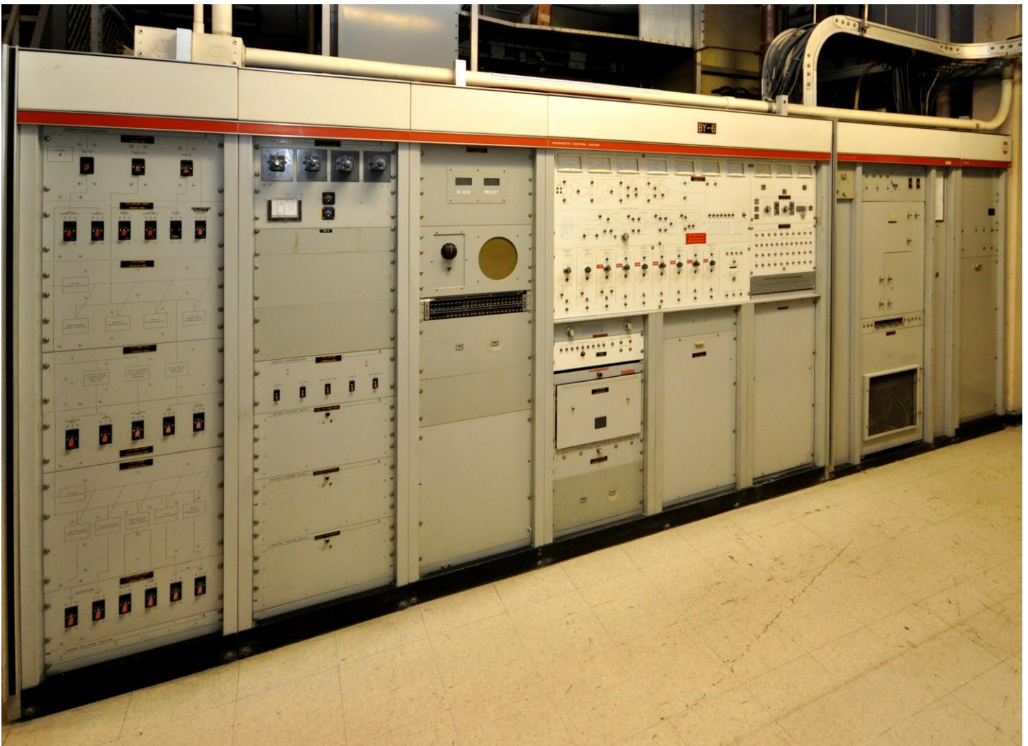
Collins Radio 821A-1, 250 KW, Transmitter
